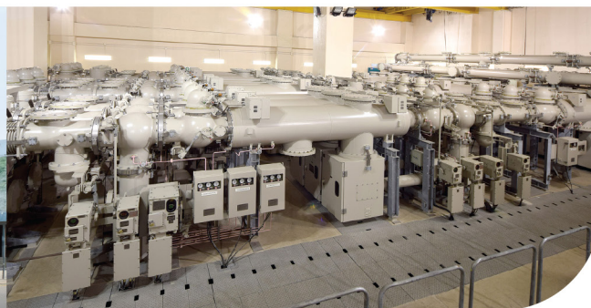
275kV Gas Insulated Switchgear 275kV 氣體絕緣開關
