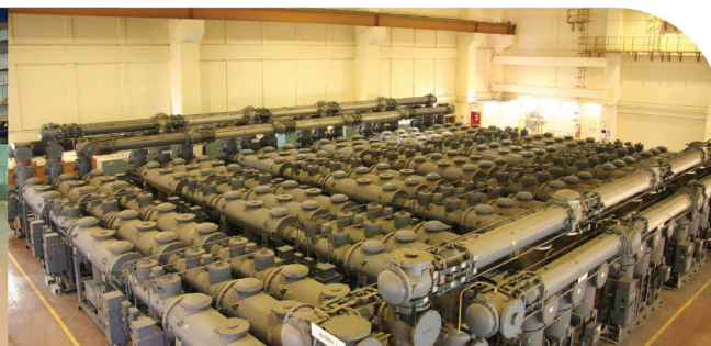
400kV Gas Insulated Switchgear 400kV 氣體絕緣開關
